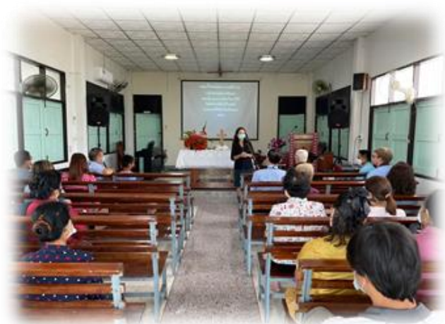
This old building was in poor condition. The ceiling and roof are failing due to
